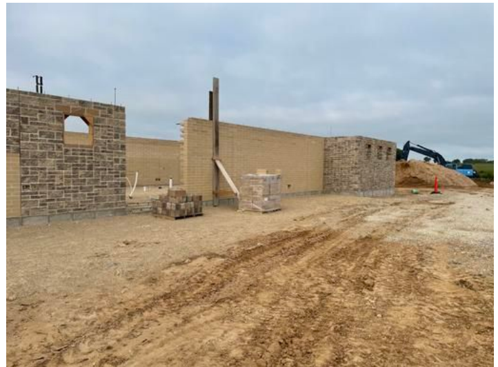
Masonry walls Bath House Taken on Jul 20, 2023, 7:50 AM CDT Added on Jul 20, 2023, 9:22 AM CDT Added by andrew gordon
