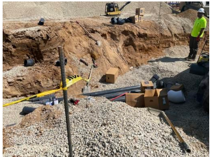
underground piping for waterslides Taken on Jul 21, 2023, 10:34 AM CDT Added on Jul 21, 2023, 11:01 AM CDT Added by andrew gordon
