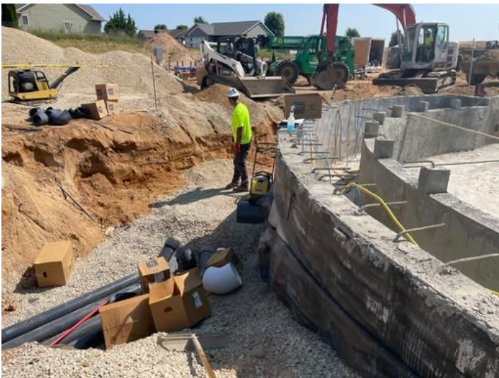
Excavating for waterslides Taken on Jul 21, 2023, 10:34 AM CDT Added on Jul 21, 2023, 11:01 AM CDT Added by andrew gordon
